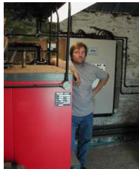
Sam with 150kW Binder Boiler
