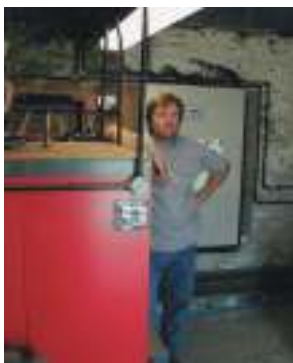
Sam next to his 150kW Binder boiler at Grascott Farm north of Okehampton
